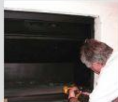
Logpan removed and a 25mm hole is drilled on the RHS of the firebox.
